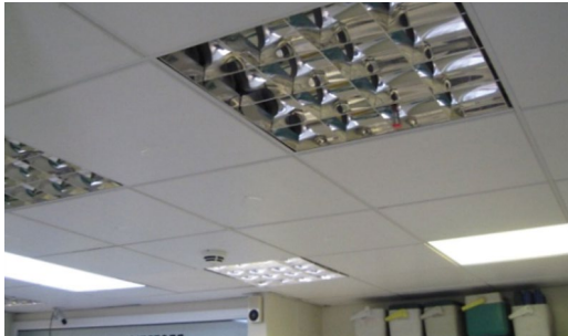
Figure 32 Inappropriate luminaires for application modular lay-in in retail
