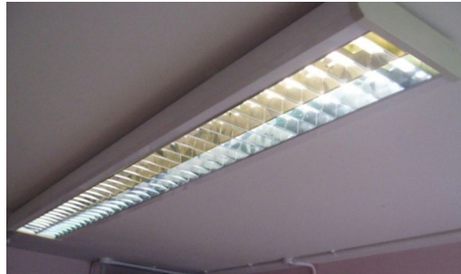
Figure 33 Poor maintenance illustrated by mixture of lamps in luminaire
